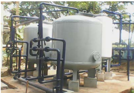
50,000 m3/hr Arsenic & Iron Removal System in Taranipur Village, Barasat, North 24 Parganas
